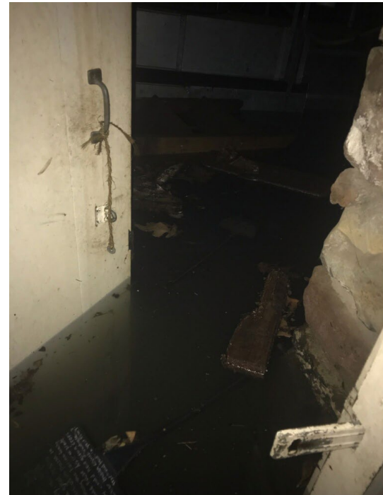
Inundation in Wyckoff House’s cellars caused by Hurricane Ida. Source: Wyckoff House Museum 2021b.
